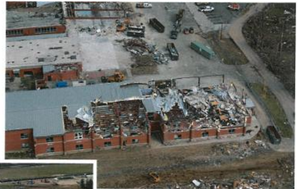
Henryville Junior Senior High School damaged by EF-4 tornado. Photo: Double D Consulting
